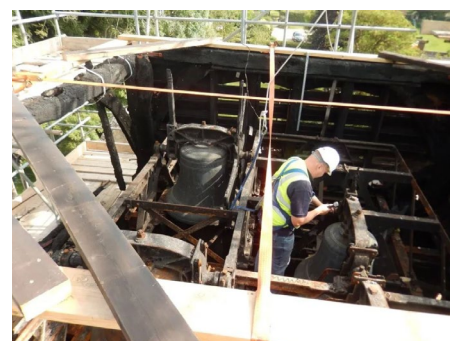
Removing the bells after the fire
